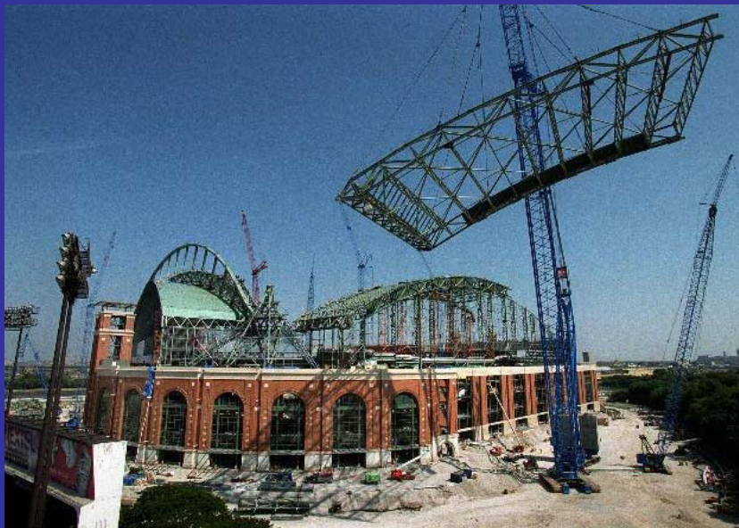
Hours before collapse of "Big Blue"
